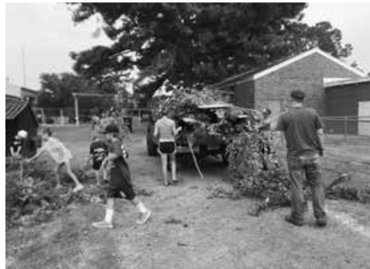
ST. MARY'S SCHOOL (NATCHITOCHE) CLEAN UP DAY. On Saturday, July 28, St. Mary's held a work day. Several parents and students came out to help work and clean up around the school. The awnings were repaired and the poles painted; windows, gutters, and sidewalks were cleaned and branches were hauled away; exercise equipment was assembled in the weight room. St. Mary's thanks those who came out to help. (To see more pictures go to www.diocesealex.org .)
