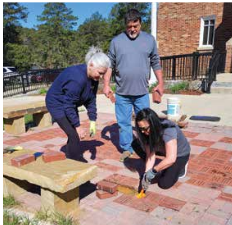
A LENTEN SEASON OF SERVICE PROJECT was performed on Saturday, Mar. 4 by Team Texada Brick Project. The team laid and set some of the memorial bricks at Maryhill Renewal Center. Team members: BH and Grace Texada, and Lori Constantino Wehrle.
