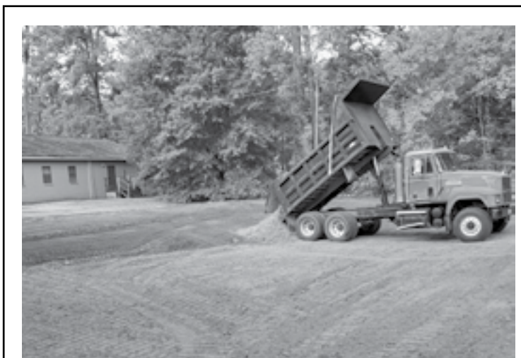
MARYHILL UPDATES. The old swimming pool adjacent to the Youth Center has been deconstructed and filled in. Plans include a renovation of the restroom building.
